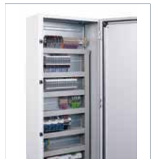
SPS control unit
